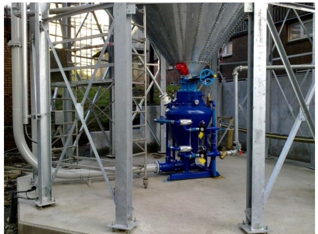
System 2 fully installed and running
