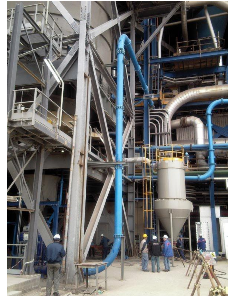
Power station boiler building – system 3
