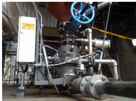
View of the installed system
