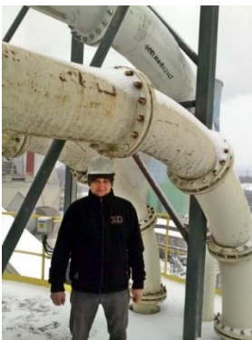
Pipe lines at the reception end
