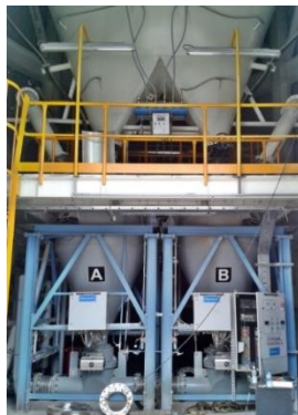
Macpump T150 installed
