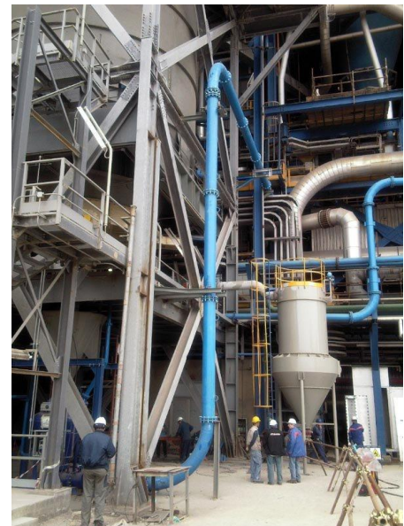
Power station boiler building – system 3
