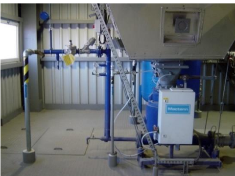
Primary vessel showing conveying air supply
