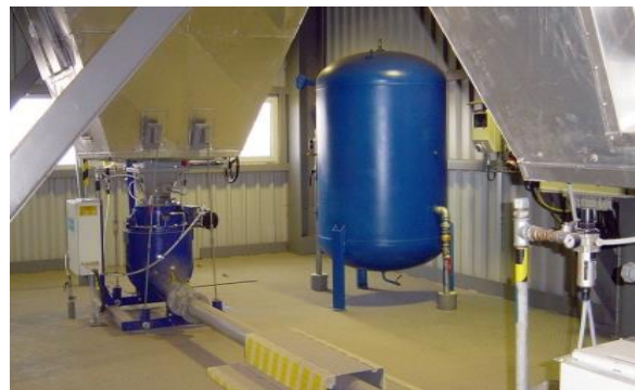
Another view of the first vessel showing the air reservoir
