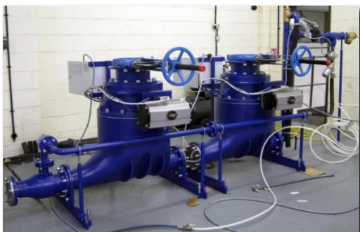
Part of system 2 during functional testing & pressure test
