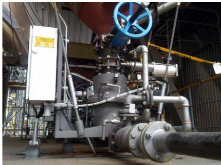
View of the installed system
