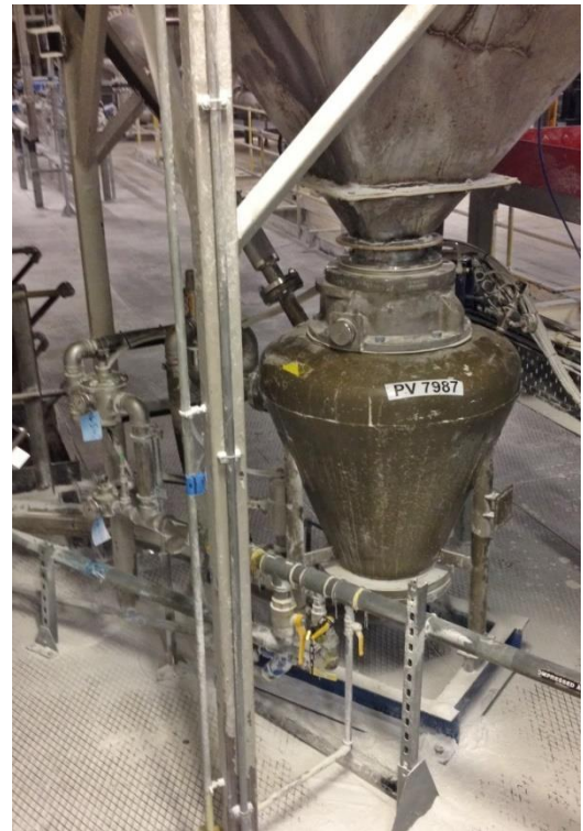
Denseveyor® installed below a feed hopper
