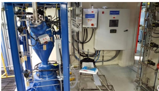
Actual installation at the research facility
